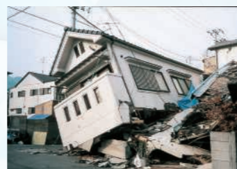
A house destroyed in the Great Hanshin-Awaji Earthquake, photographed by Professor Kenji Miyazawa
